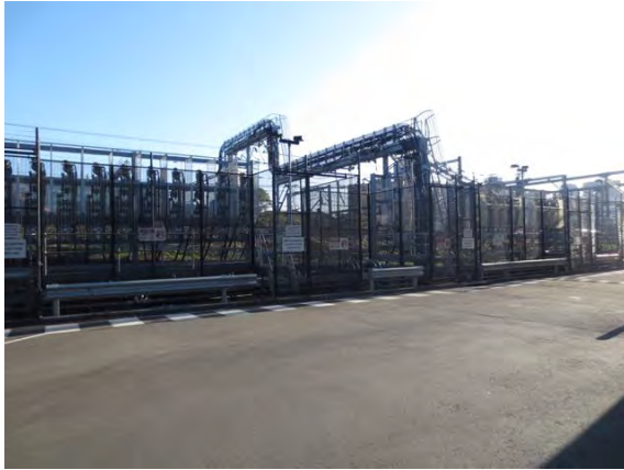
Figure 50: Perimeter fence and cable gantry.
