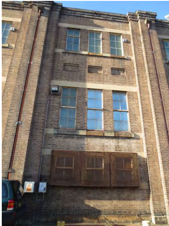
Figure 40: West elevation of Prince Alfred Substation. Note brick piers and corbelled top. The building has a strong vertical emphasis.
