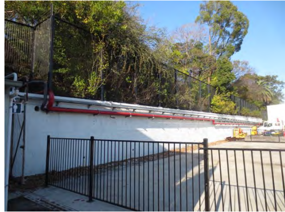
Figure 51: Retaining wall and embankment along eastern boundary of site towards Prince Alfred Park.
