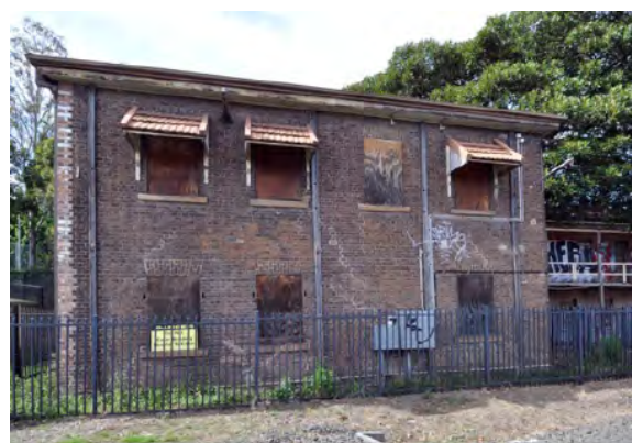
Figure 55: Former District Engineer's Office west façade, fenced off and boarded up.
