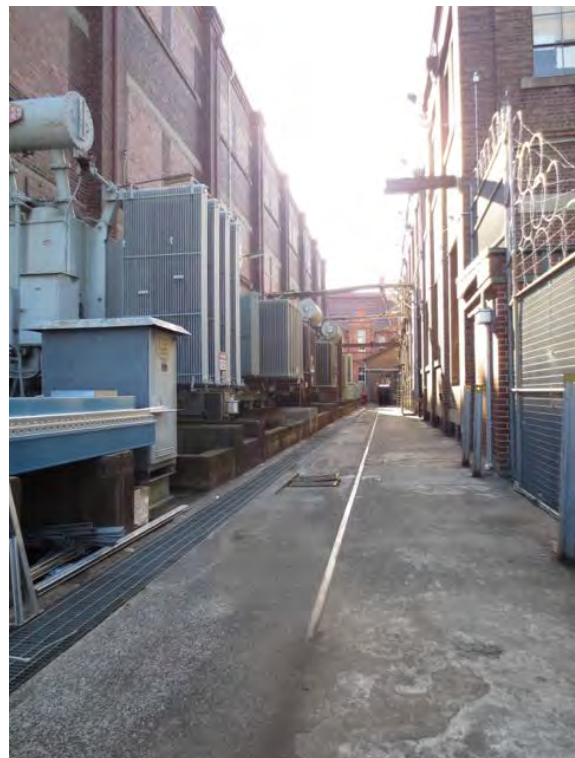
Figure 43: Looking north with Prince Alfred substation on the left and Switching House on the right.
