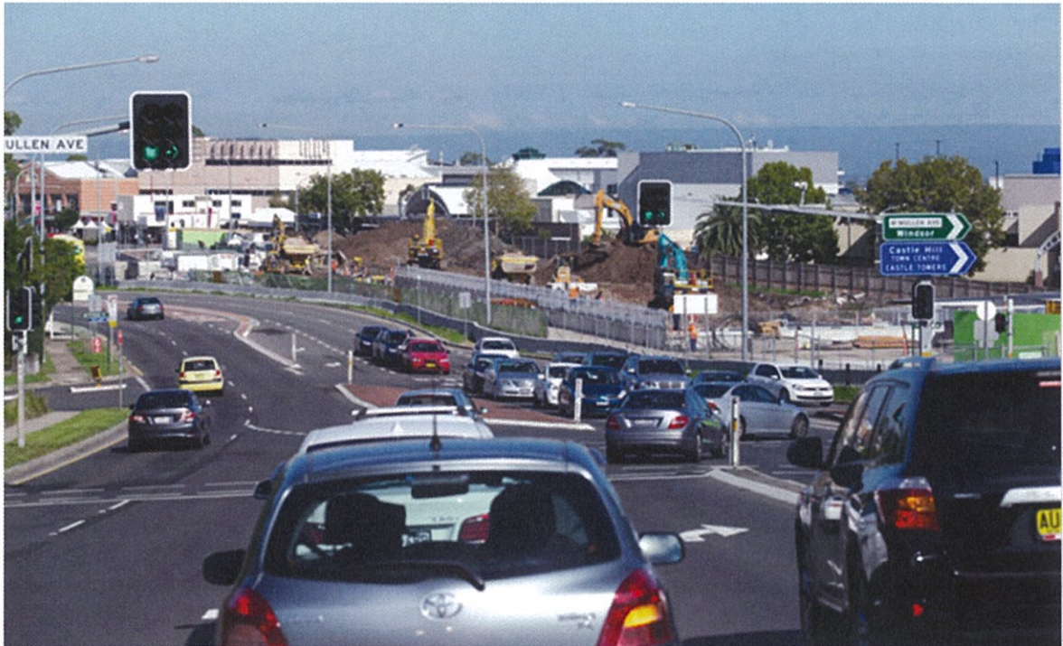
Figure 5 – Castle Hill Station Site at the Intersection of Old Northern Rd and McMullen Ave
